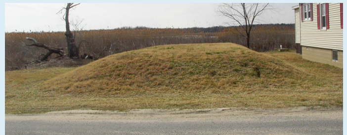
As sea level rises, the water table rises as well, which can prevent ordinary septic systems from working properly. The owner of this house in Pickering Beach responded by shifting to a mounds-based system, which provides the required separation between the drain field and the water table. © James G. Titus; used by permission.
