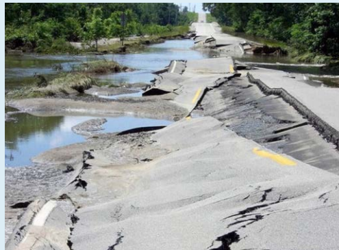
Flooding of the Cedar River in 2008 damaged this section of U.S. Highway 6 east of Atalissa. Credit: Iowa Department of Transportation.
