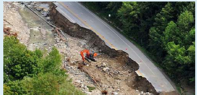
In 2011, Hurricane Irene caused major flooding and damaged infrastructure across Vermont, including this section of Route 107 in Stockbridge. Heavy storms are becoming more common as a result of climate change. Credit: Vermont Agency of Transportation.
